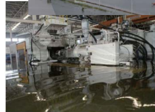
Damage to machinery due to flooding
